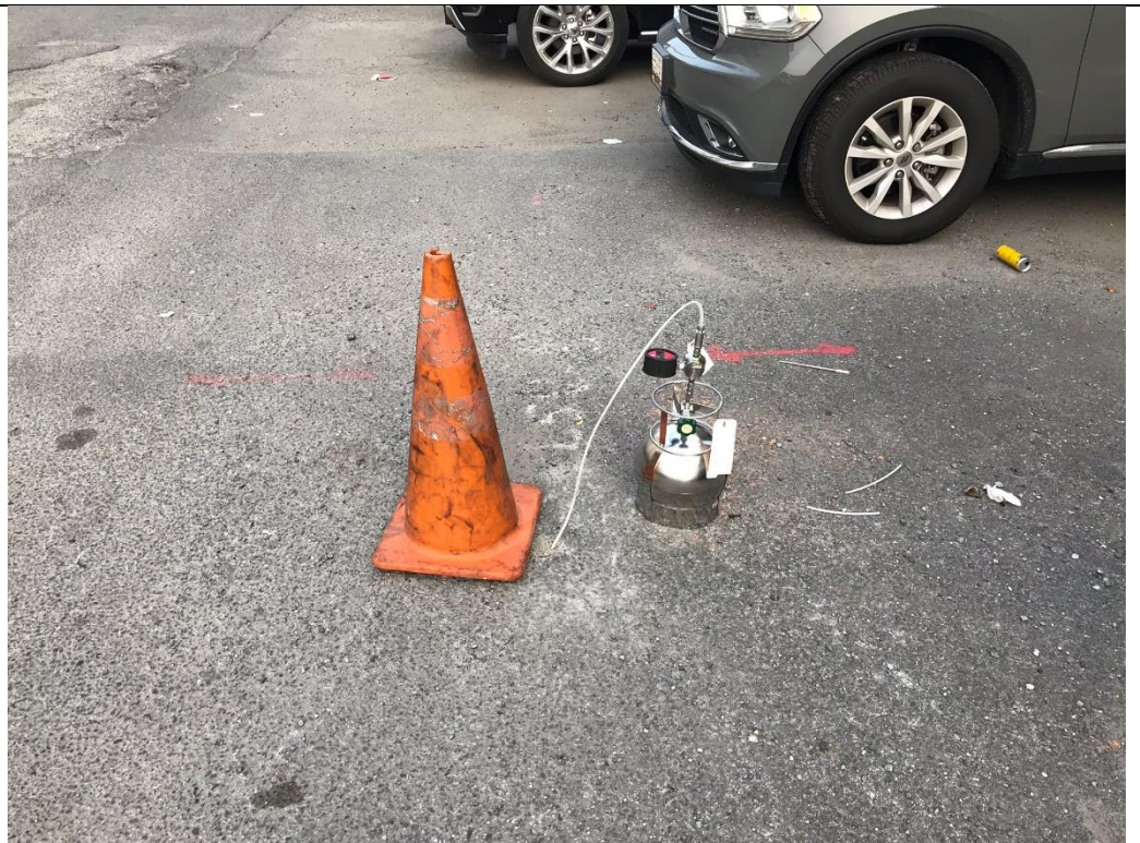
Photo 2 – Collection of LSV-14 soil vapor sample, facing west.
