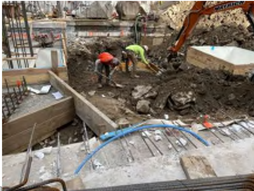
Photo 2: Mayrich removing chipped bedrock from the central part of the site (facing west).
