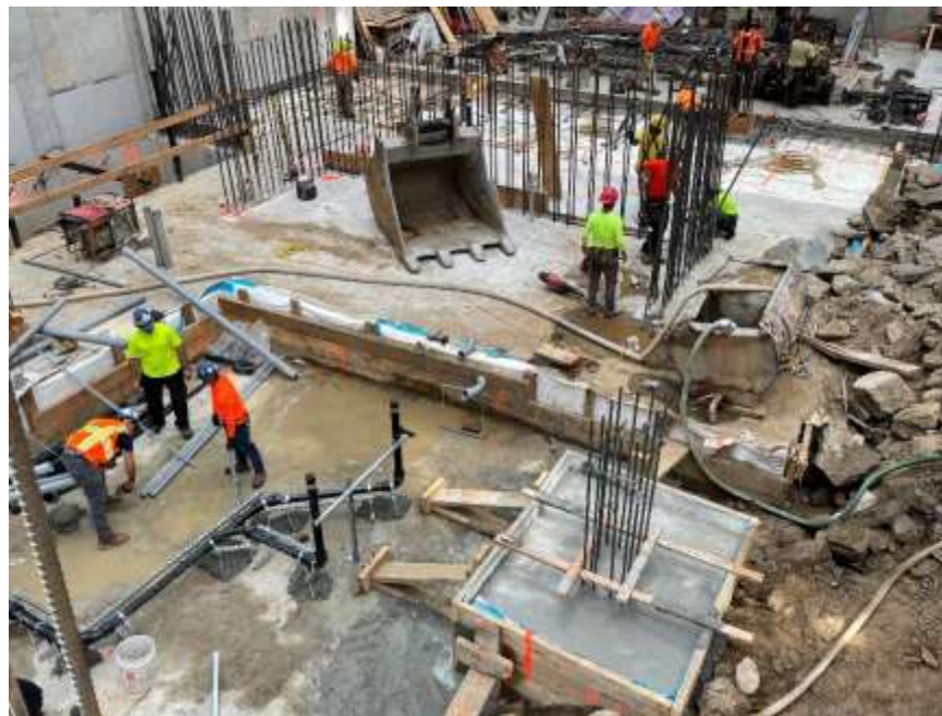
Photo 14: View of the on-site segment of the dewatering system, facing southeast. Taken on 08/08/2022
