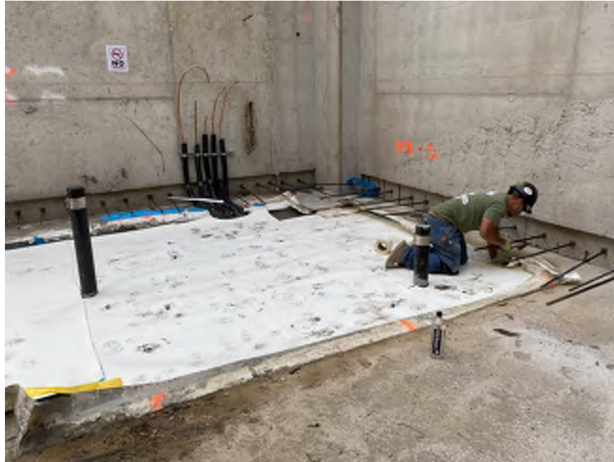
Photo 1: View of Mayrich installing waterproofing in the northeastern part of the site (facing northeast).
