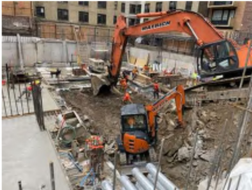
Photo 2: View of Mayrich removing chipped bedrock from the central part of the site (facing southwest).
