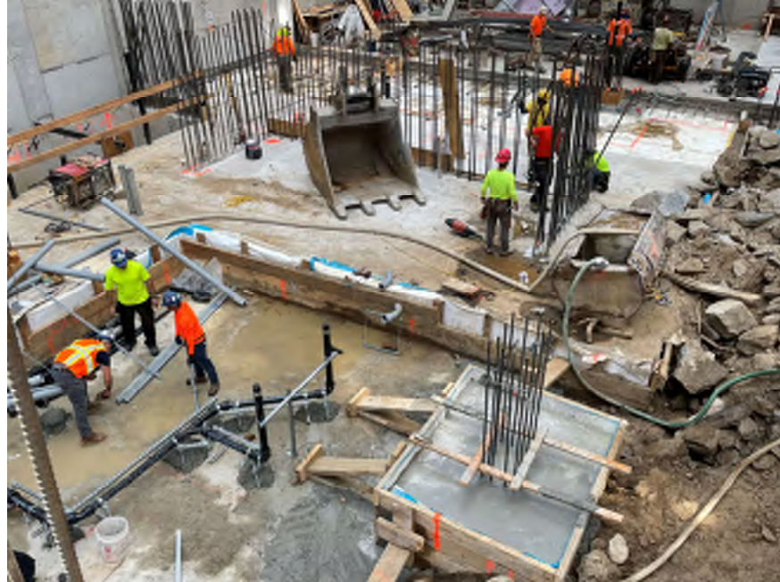
Photo 1: View of the on-site segment of the dewatering system (facing southeast).
