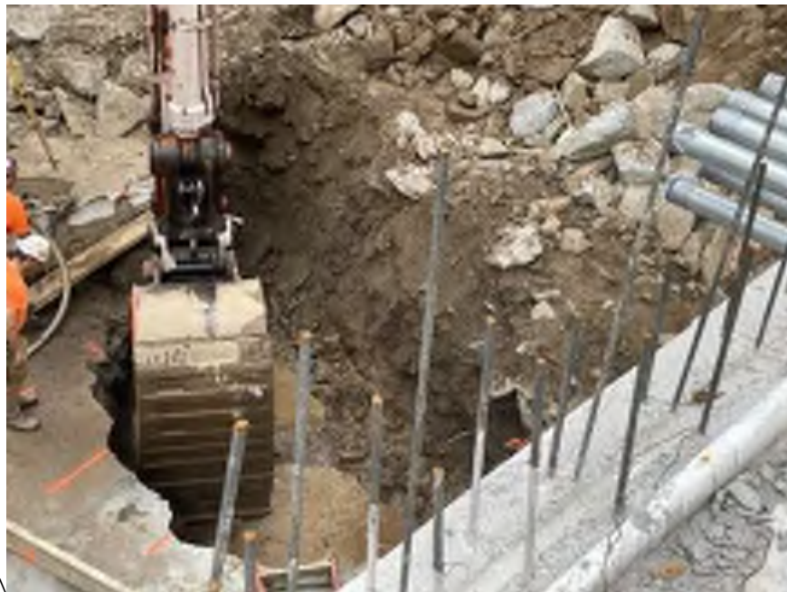
Photo 2: Mayrich removing chipped bedrock in the northeastern part of the site (facing south).
