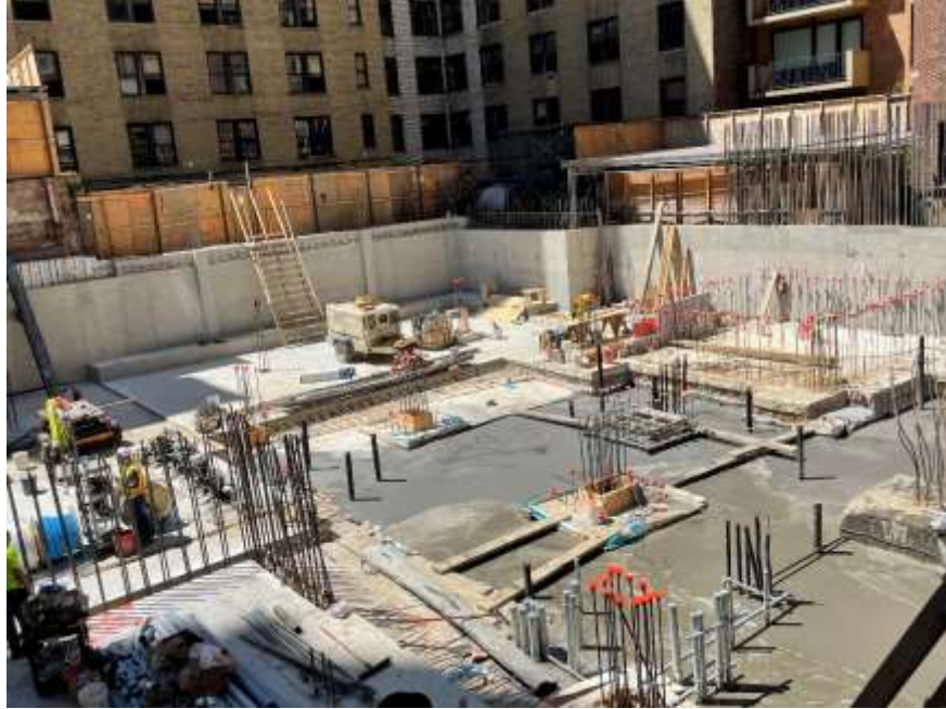
Photo 17: General view of the site with completed rat slab, facing southwest. Taken on 08/19/2022
