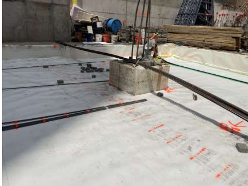
Photo 1: View of Mayrich installing waterproofing in the southwestern part of the site (facing west).
