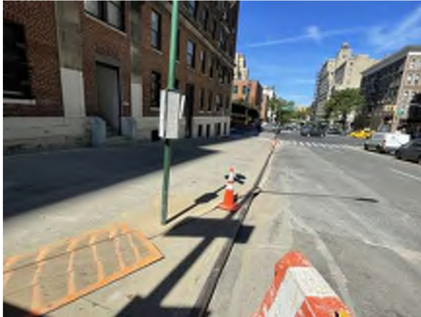
Photo 1: View of off-site components of the site's dewatering system (facing west). Taken 08/16/2022
