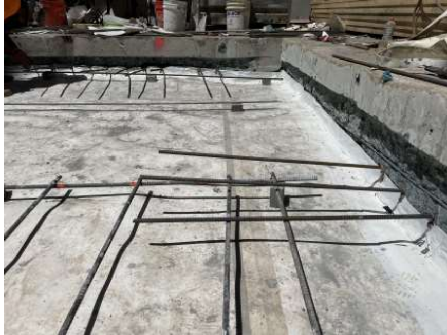
Photo 1: View of area Mayrich installed waterproofing in the southwestern part of the site (facing west).
