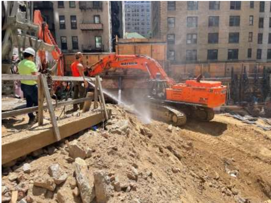
Photo 10: View of Mayrich apply water to mitigate dust on the central part of the site, facing south. Taken on 06/20/2022
