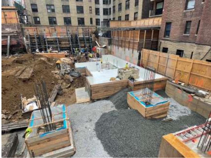
Photo 9: View of the area Mayrich temporarily backfilled with 0.75-inch stone to use as a construction entrance in the northwestern part of the site, facing south. Taken on 6/16/2022
