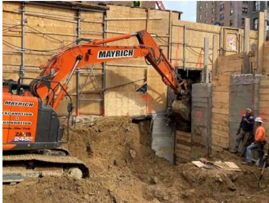
Photo 7: View of Mayrich installing lagging in northwestern part of site, facing west. Taken on 05/26/2022
