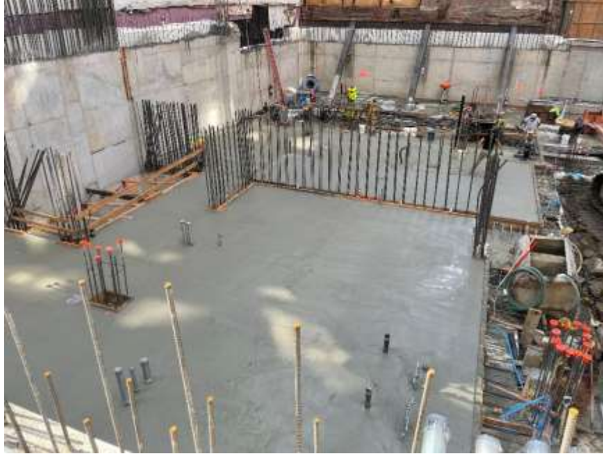
Photo 15: View of concrete rat slab poured in the eastern part of the site, facing south. Taken on 08/08/2022
