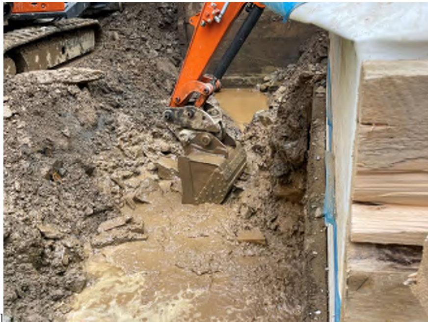
Photo 2: View of Mayrich excavating native soil from the northwestern part of the site (facing south).
