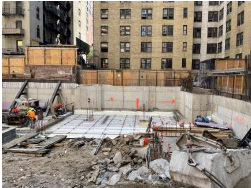
Photo 2: General view of current site conditions in the southwestern part of the site (facing south).
