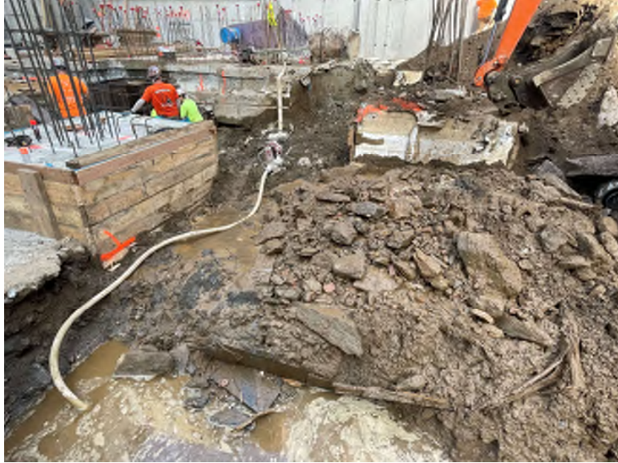
Photo 1: View of on-site components of the site's dewatering system in northwestern part of the site (facing west).
