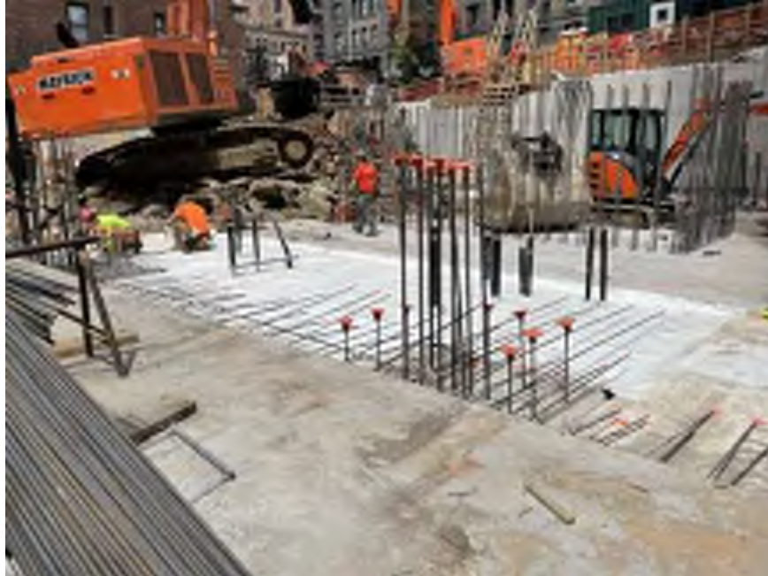
Photo 1: View of area Mayrich installed waterproofing in the eastern part of the site (facing northwest).
