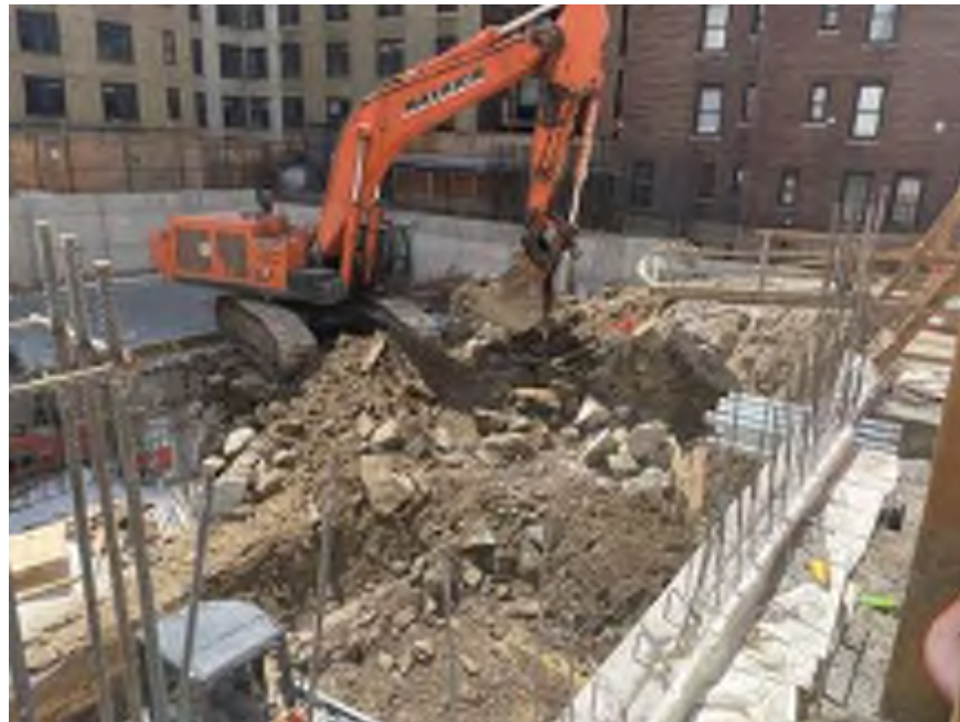
Photo 2: Mayrich excavating chipped bedrock in the northeastern part of the site (facing southwest).
