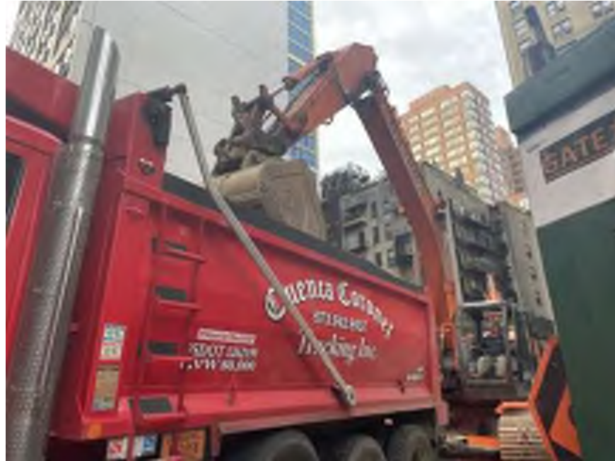
Photo 1: View of Mayrich off-loading C&D and chipped bedrock from the temporary trucking ramp in the northwestern part of the site (facing southwest).
