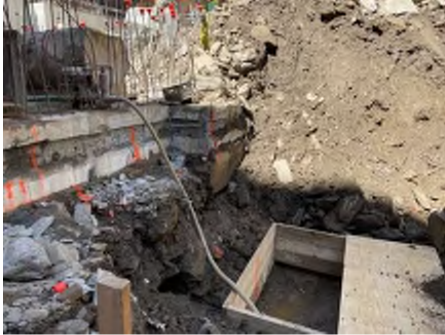
Photo 1: View of Mayrich dewatering in the central part of the site (facing north).
