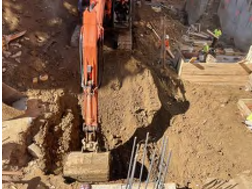
Photo 1: Mayrich excavating non-hazardous historic fill and native soil in the northwestern part of the site (facing south).
