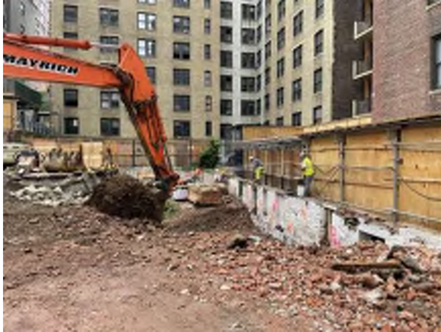
Photo 1: Mayrich using dust suppression during removal of C&D debris in the southwestern part of the site (facing south).
