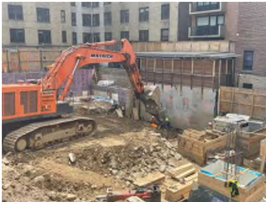
Photo 2: Mayrich excavating native soil along the western site boundary of the site for underpinning installation (facing southwest).
