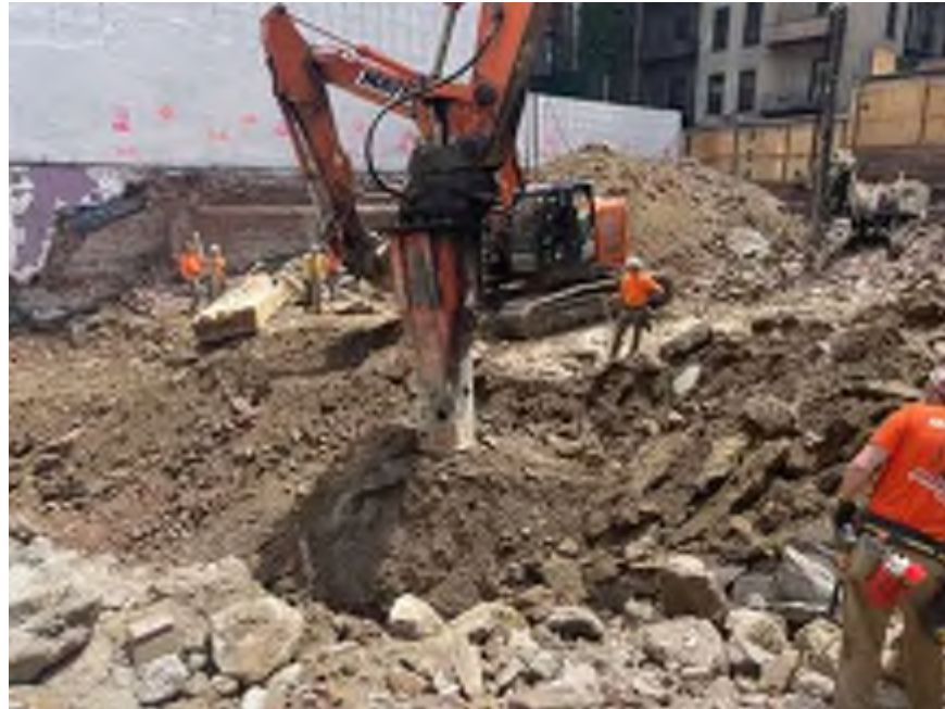
Photo 1: Mayrich applying dust suppression while breaking concrete in the northern part of the site (facing southeast).
