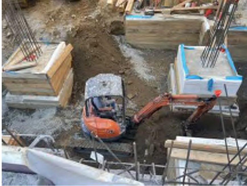
Photo 1: View of Mayrich excavating native soil from the northwestern part of the site (facing south).
