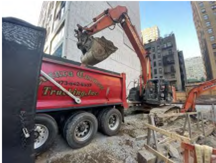
Photo 1: Mayrich exporting non-hazardous fill and native soil for off-site disposal (facing south)
