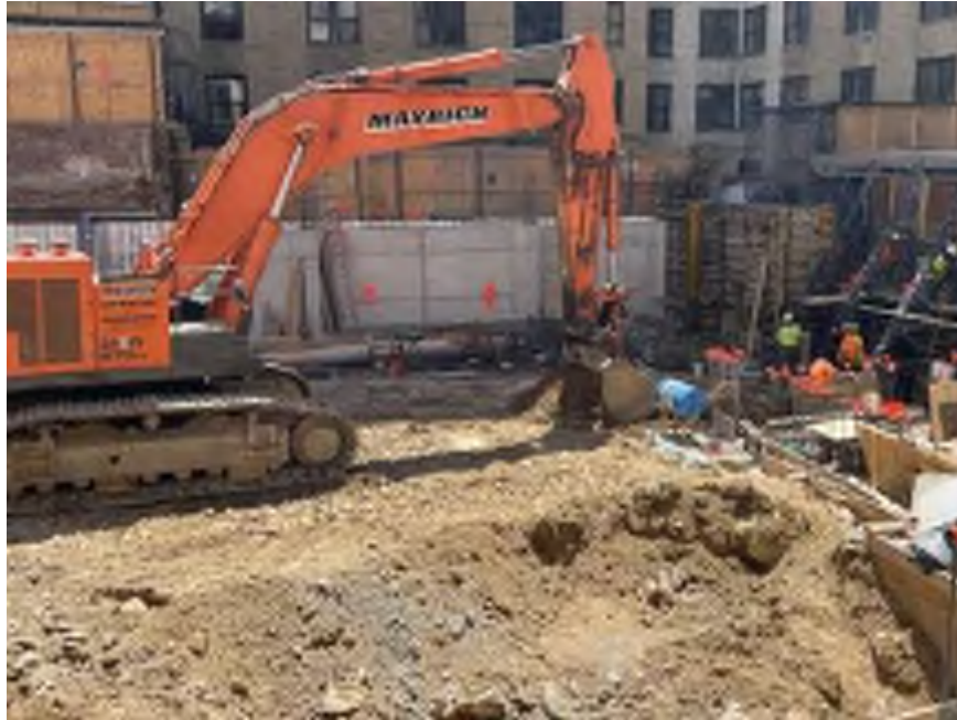
Photo 1: Mayrich excavating non-hazardous fill and native soil from the southwestern part of the site (facing south)
