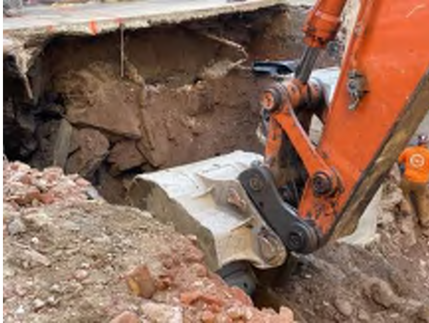
Photo 1: Mayrich excavating non-hazardous historic fill and native soil in the northern part of the site for SOE installation (facing north).
