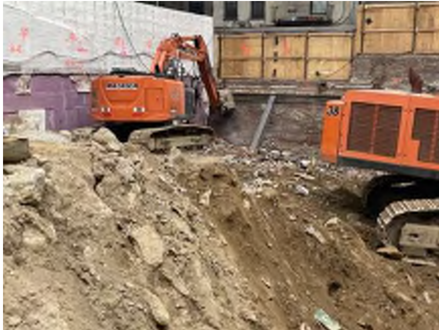
Photo 2: Mayrich removing C&D debris in the southwestern part of the site (facing south).
