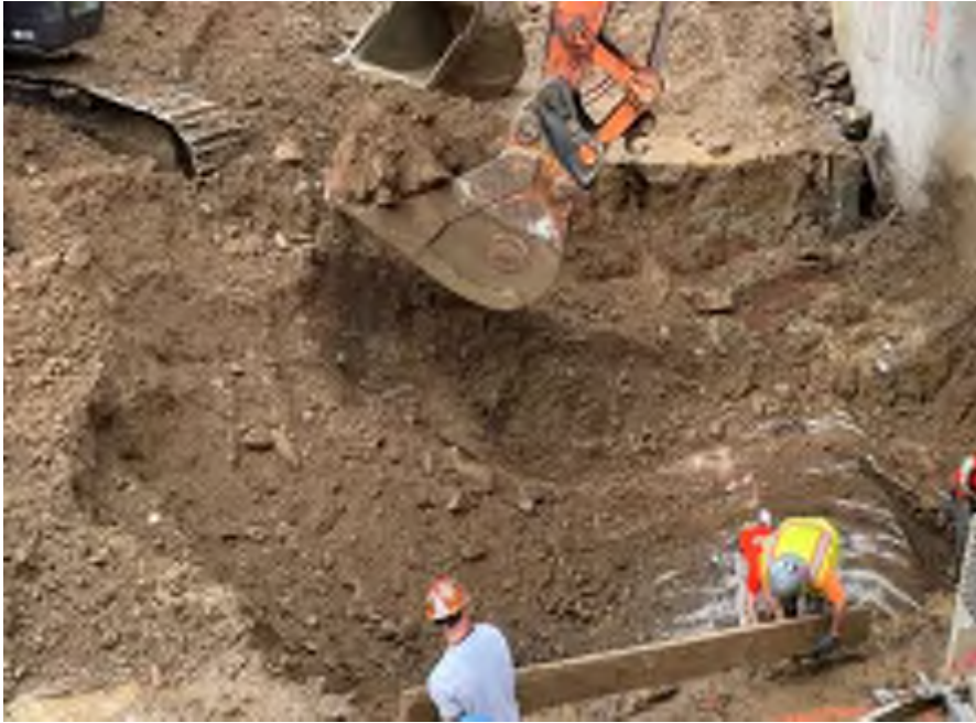
Photo 1: Mayrich excavated non-hazardous historic fill and native soil to bedrock in the northwestern part of the site (facing southwest).
