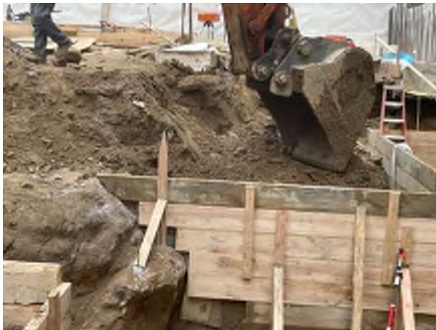
Photo 2: Mayrich excavating native soil in the western part of the site (facing south).
