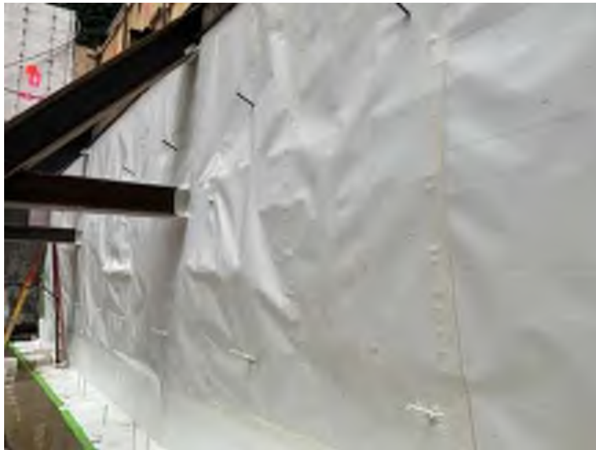
Photo 2: General view of waterproofing installed along the southern boundary on the site (facing southeast).
