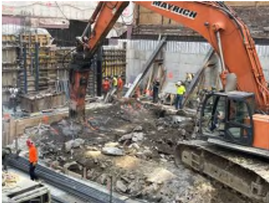
Photo 1: View of Mayrich using dust suppression while chipping bedrock in the southeastern part of the site (facing southeast).
