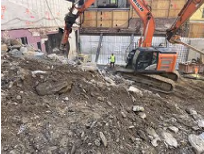
Photo 2: Mayrich using dust suppression while breaking concrete in the southeastern part of the site (facing south).
