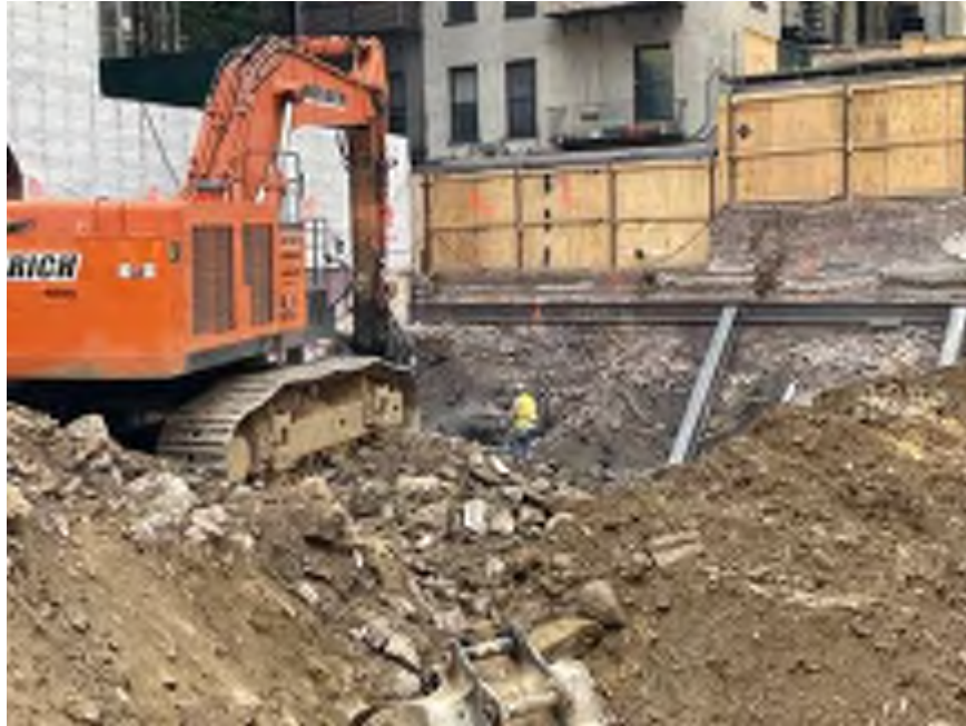
Photo 1: Mayrich using dust suppression while chipping bedrock in the southeastern part of the site (facing south)
