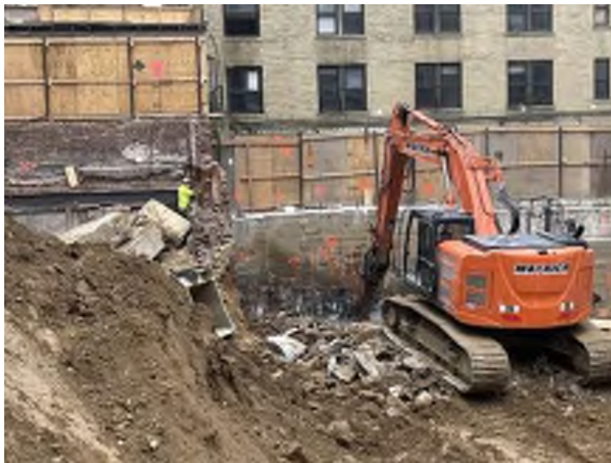
Photo 2: Mayrich applying dust suppression during bedrock chipping in the southwest part of the site (facing west).
