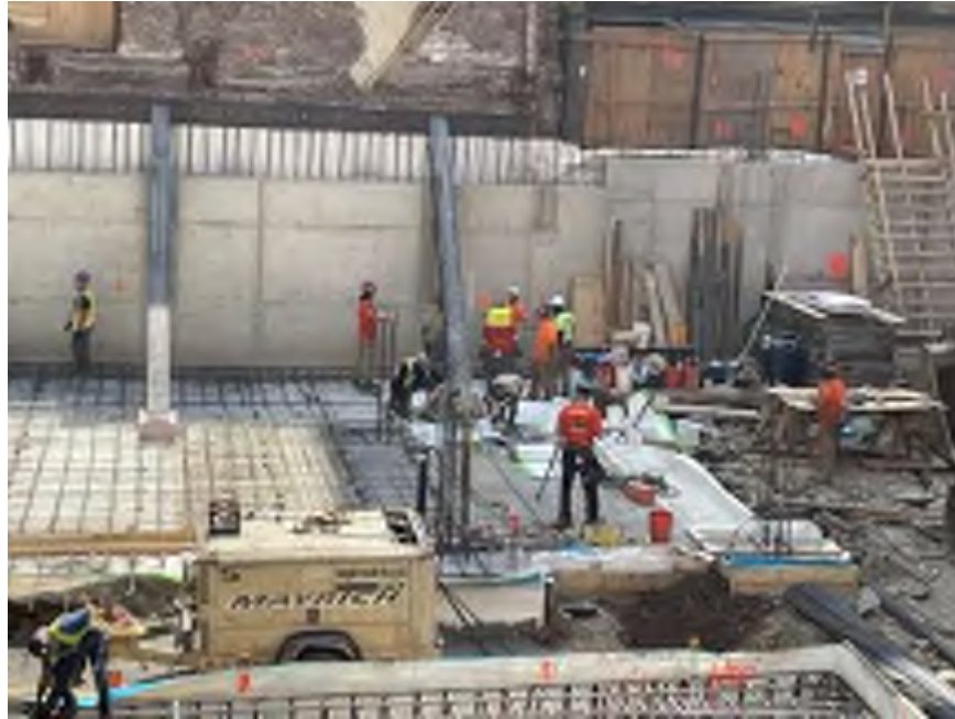
Photo 1: View of Mayrich installing waterproofing for the building's slab in the southern part of the site (facing south).
