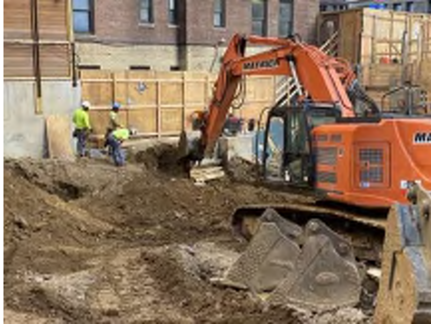
Photo 1: Mayrich excavating non-hazardous historical fill and native soil in the southwestern part of the site (facing northwest).
