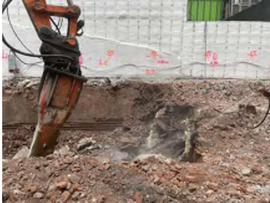
Photo 1: Mayrich applying water to the work area in the northeastern part of the site (facing east).
