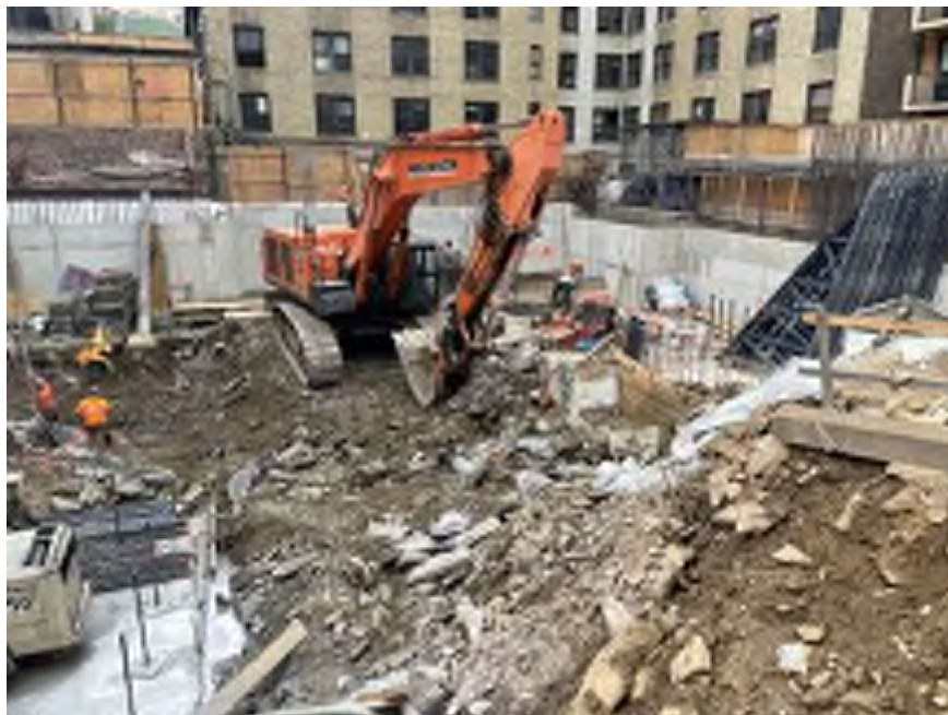
Photo 2: View of Mayrich grading chipped bedrock in the southwestern part of the site (facing south).
