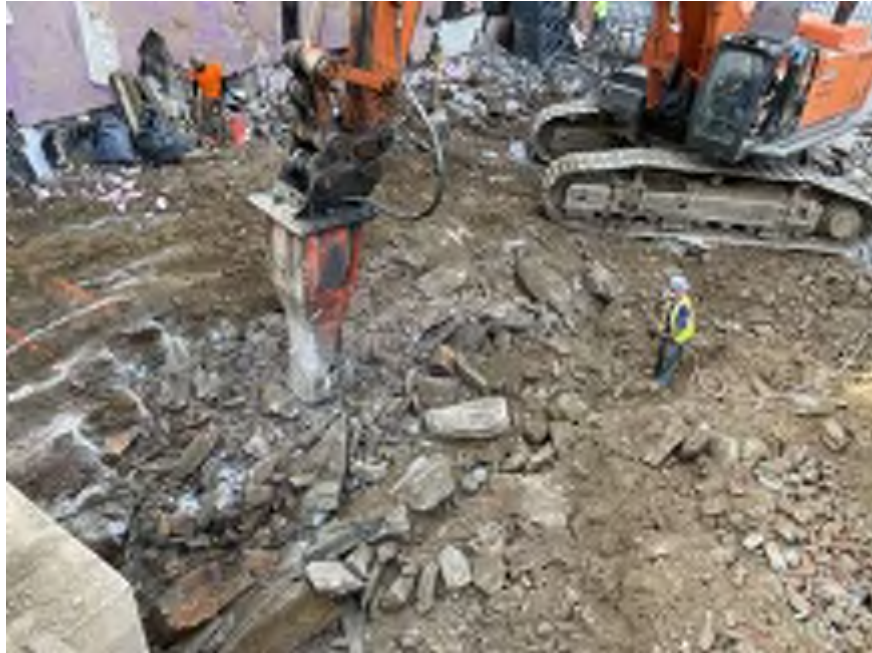
Photo 1: View of Mayrich using dust suppression while chipping bedrock in the northeastern part of the site (facing east).
