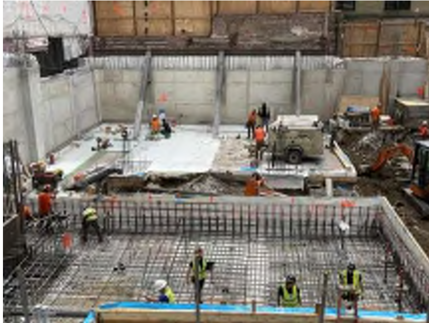
Photo 1: View of Mayrich installing waterproofing for the building's east mat in the southeastern part of the site (facing south).
