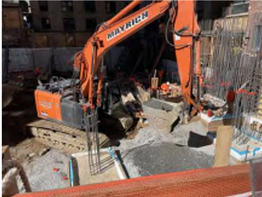
Photo 1: Mayrich excavating 0.75-inch stone in the northwestern part of the site (facing southwest)
