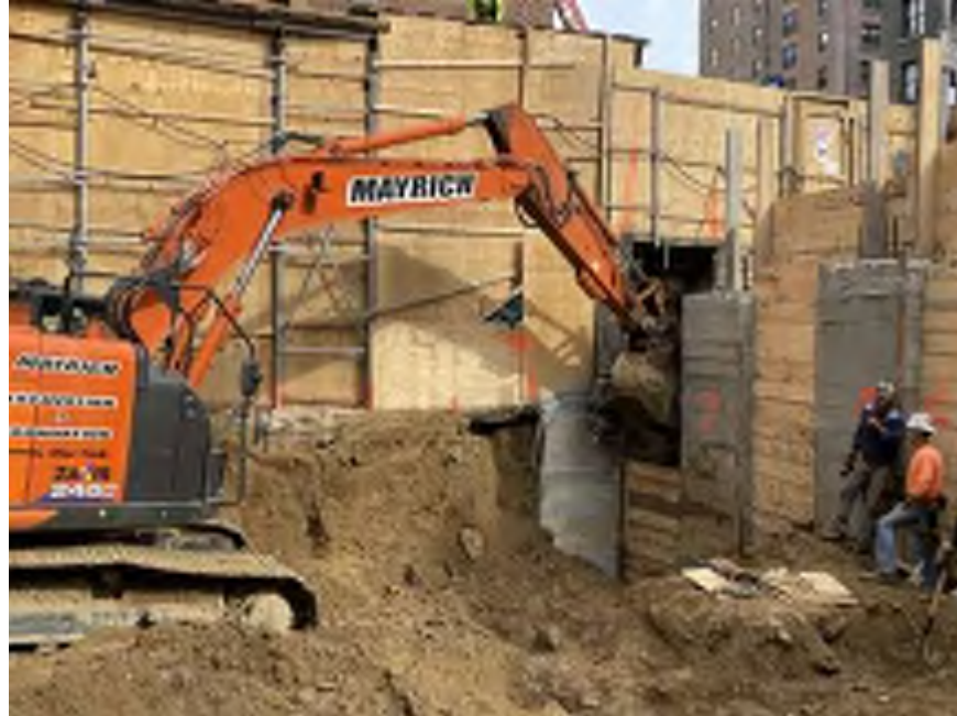
Photo 1: Mayrich excavating non-hazardous historical fill and native soil along the northwestern boundary of site (facing west).
