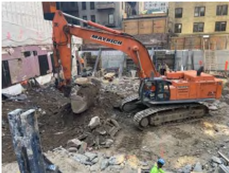
Photo 2: Mayrich removing previously backfilled C&D debris and chipped bedrock in the northeastern part of the site (facing south).
