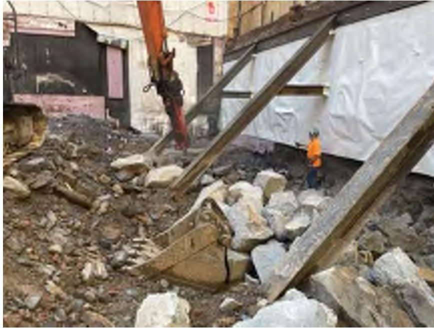
Photo 1: Mayrich using dust suppression while breaking concrete in the southeastern part of the site (facing east).
