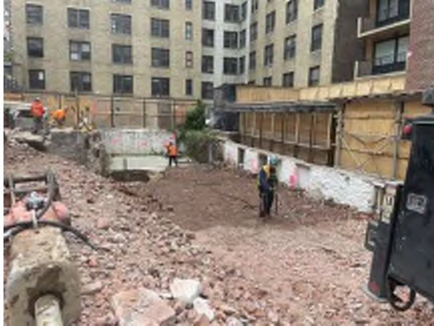
Photo 1: Mayrich applying water to the work area in the western area of site (facing south).
