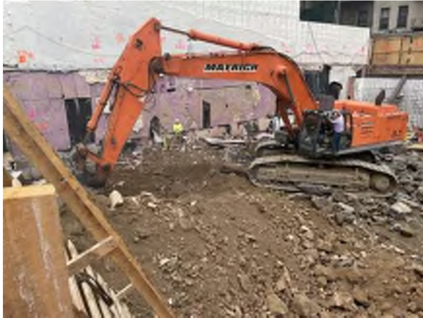
Photo 2: View of Mayrich excavating non-hazardous historic fill in the northeastern part of the site (facing southeast).
