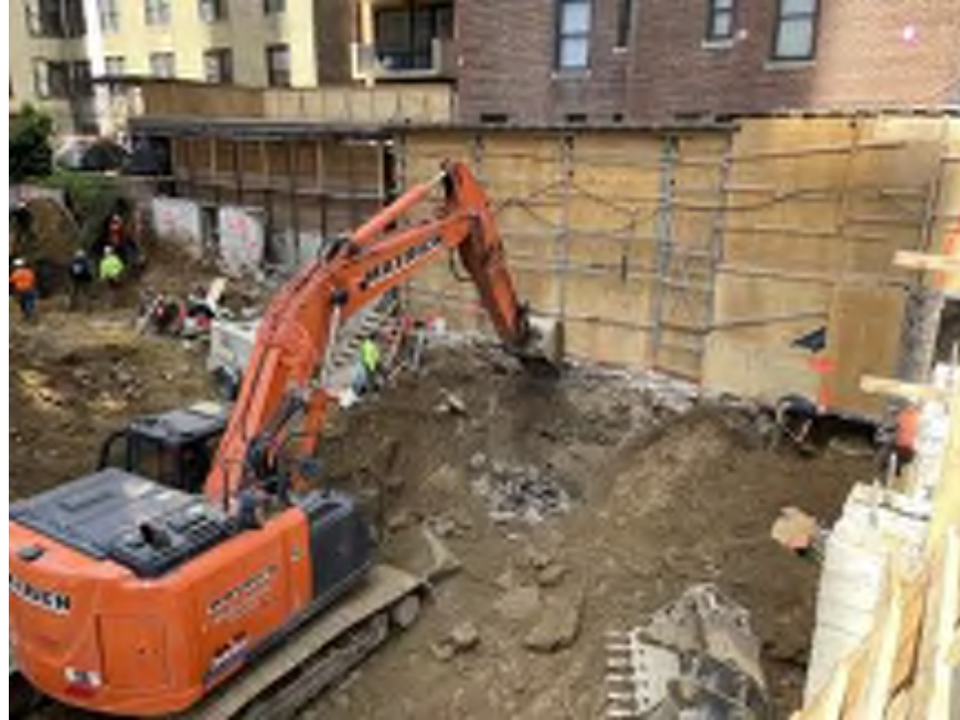
Photo 1: Mayrich excavating non-hazardous historical fill and native soil along the northwestern area of site (facing west).
