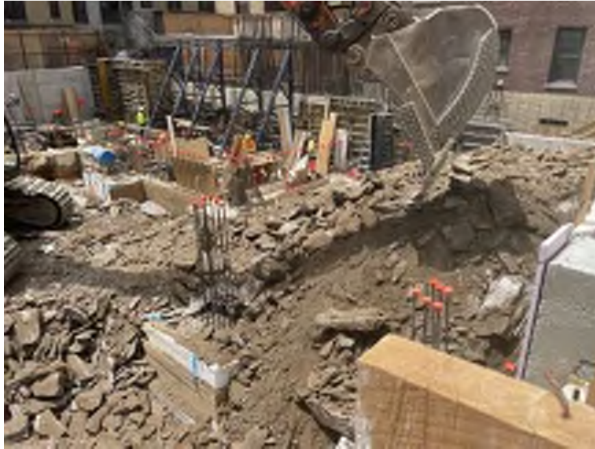
Photo 2: General view of Mayrich stockpiling chipped bedrock in the northwestern part of the site to use as a temporary equipment ramp (facing south).
