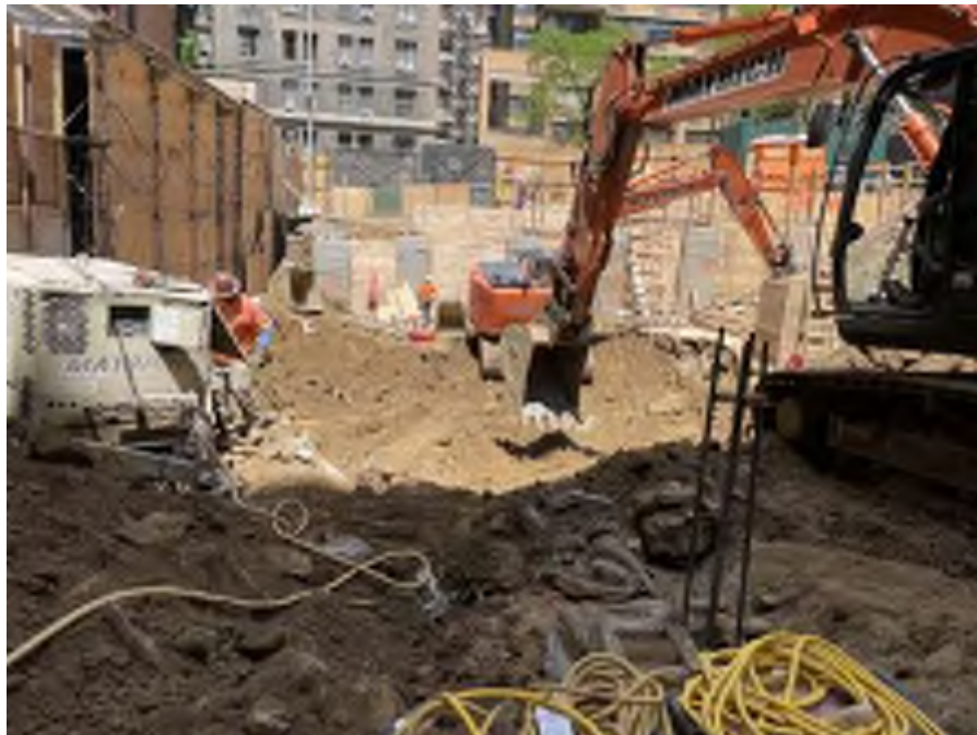
Photo 2: Mayrich grading soil in the north-central part of the site (facing east)
