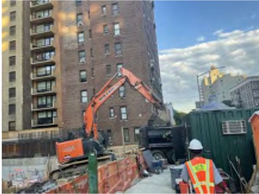
Photo 1: View of Mayrich exporting C&D and chipped bedrock for off-site disposal (facing west)
