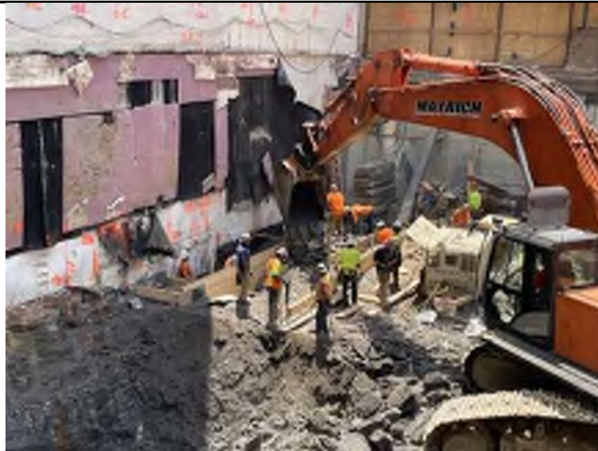
Photo 1: View of Mayrich temporary backfilling with chipped bedrock to support formwork in the southeastern part of the site (facing west)
