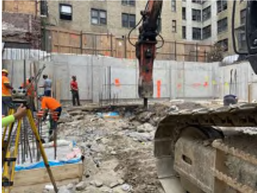
Photo 1: Mayrich using dust suppression while chipping bedrock in the southwestern part of the site (facing south).
