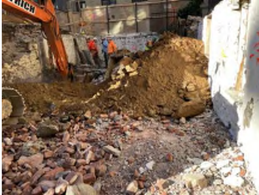
Photo 1: Mayrich excavating non-hazardous historic fill and native soil in the southwestern part of the site (facing south)
