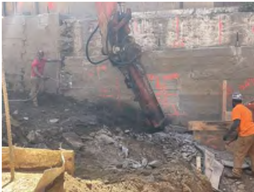
Photo 2: Mayrich applying dust suppression during bedrock chipping in the southwest part of the site (facing south).
