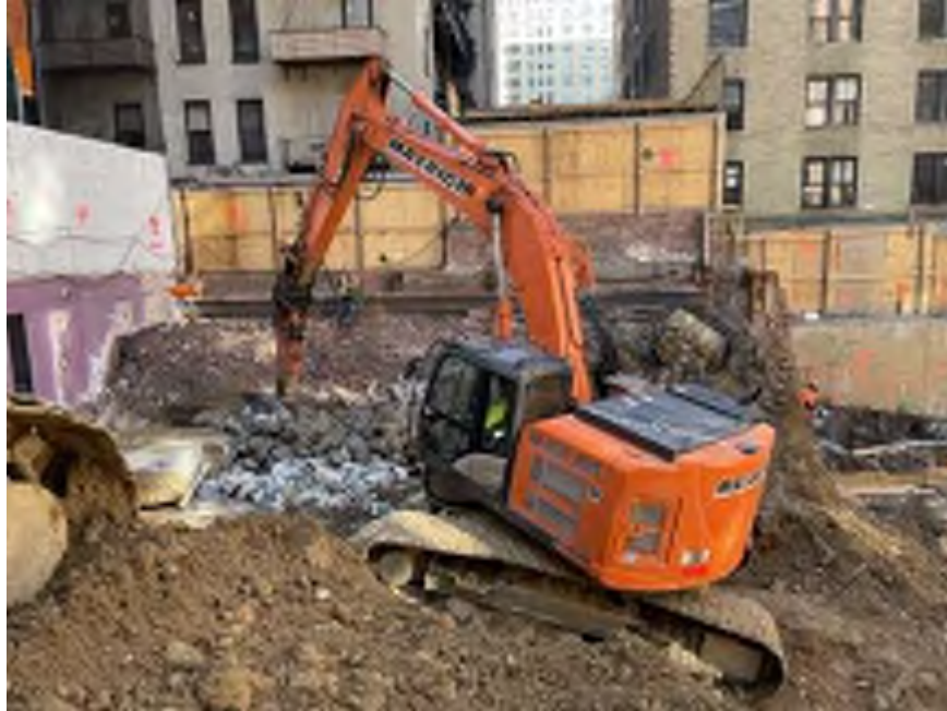
Photo 2: Mayrich applying dust suppression while breaking concrete in the southeastern part of the site (facing south).
