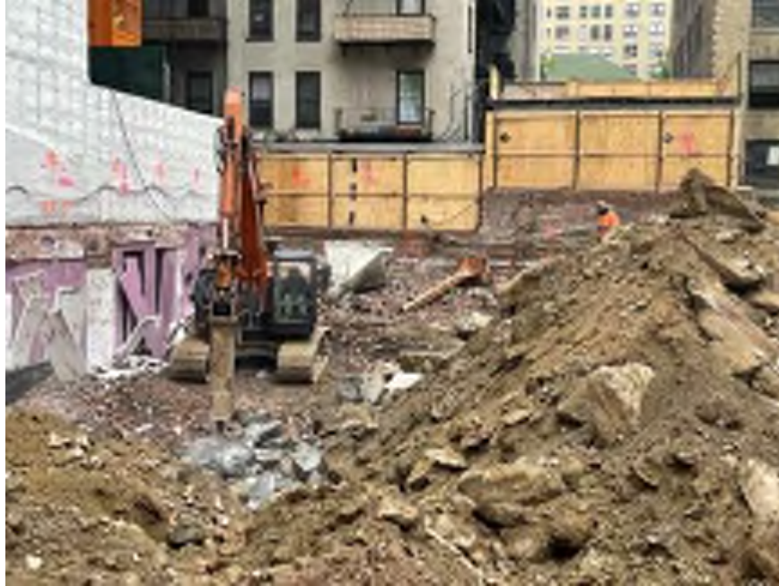
Photo 1: Mayrich using dust suppression while breaking concrete slab in the southeastern part of the site (facing south).
