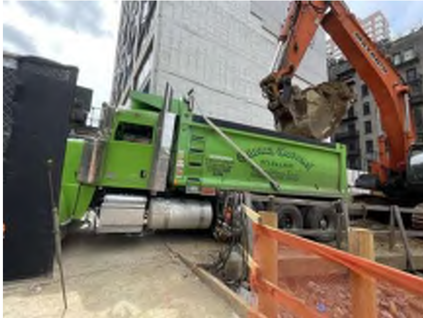
Photo 1: Mayrich exporting non-hazardous historic fill and native soil for off-site disposal (facing east).
