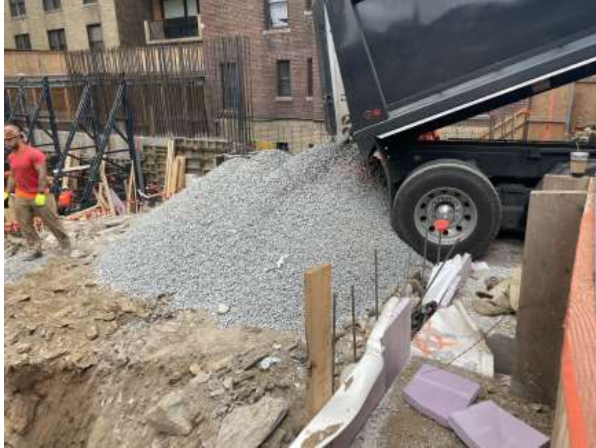
Photo 1: Mayrich importing 0.75-inch stone to be used as a temporary trucking track pad (facing west)
