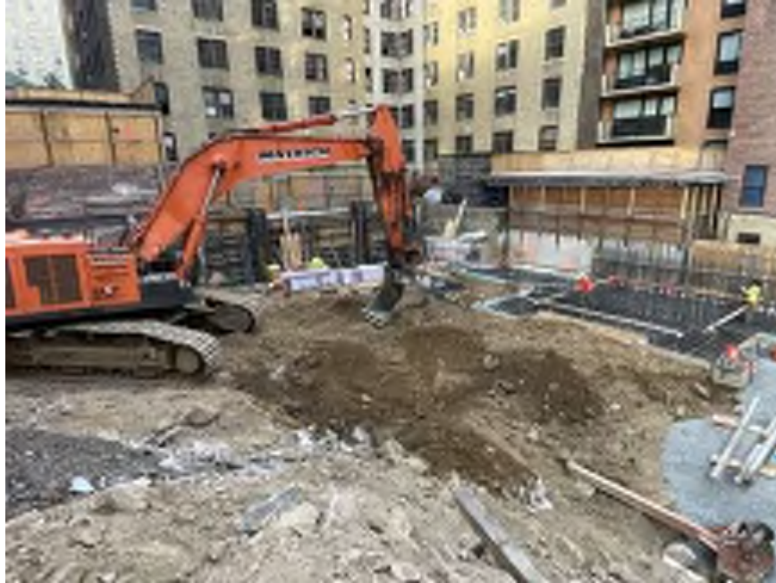
Photo 1: Mayrich grading non-hazardous historic fill in the northcentral part of the site (facing southwest).
