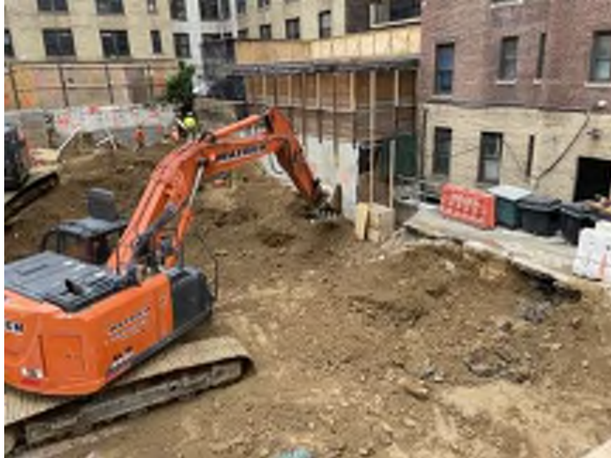
Photo 1: Mayrich excavating non-hazardous historical fill and native soil along the western boundary of site (facing southwest).
