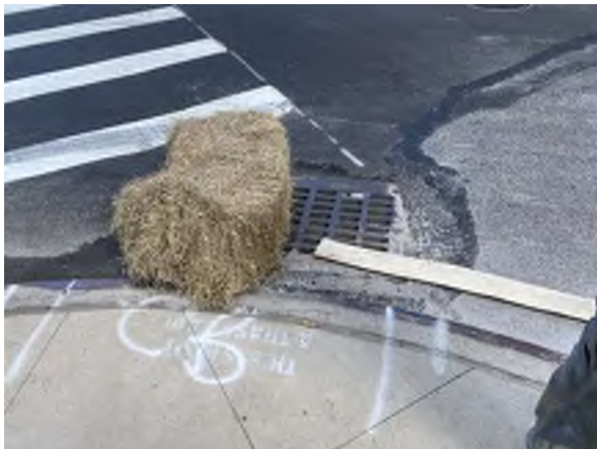
Photo 2: View of Mayrich discharging groundwater to the catch basin located at the corner of West 96 th Street and West End Avenue in accordance with the NYCDEP temporary discharge permit (facing northwest).
