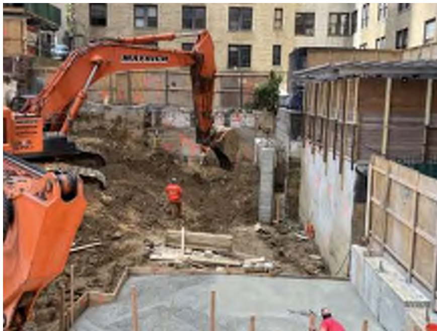
Photo 2: Mayrich excavating non-hazardous historic fill and native soil in the southwestern part of the site (facing south).
