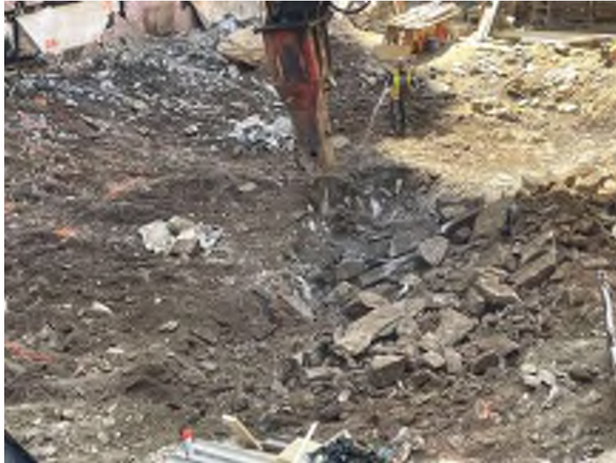
Photo 1: Mayrich using dust suppression while chipping bedrock in the central part of the site (facing south).
