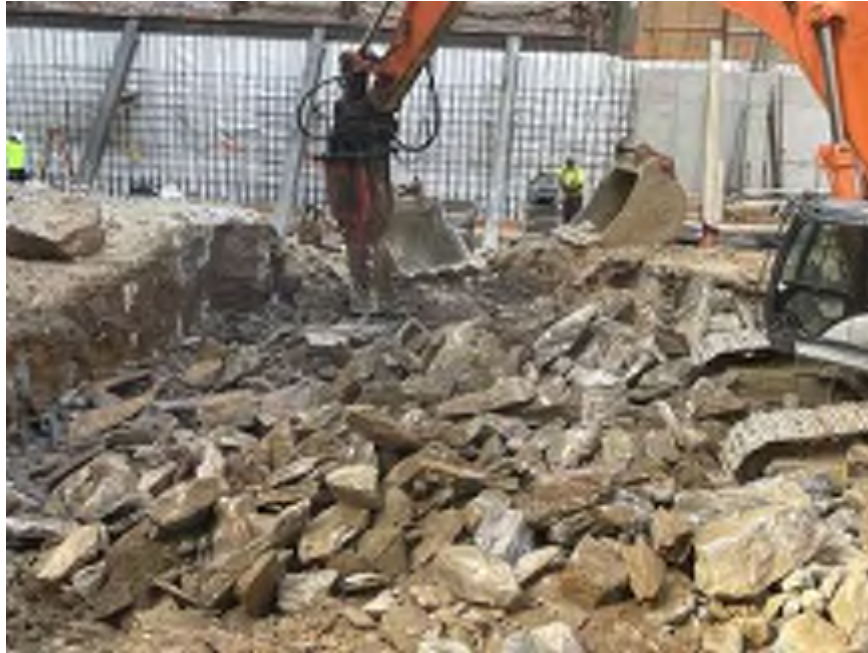
Photo 1: Mayrich using dust suppression while chipping bedrock in the central part of the site (facing south).
