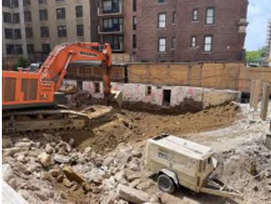
Photo 1: Mayrich excavating non-hazardous historical fill and native soil along the western part of the site (facing west).
