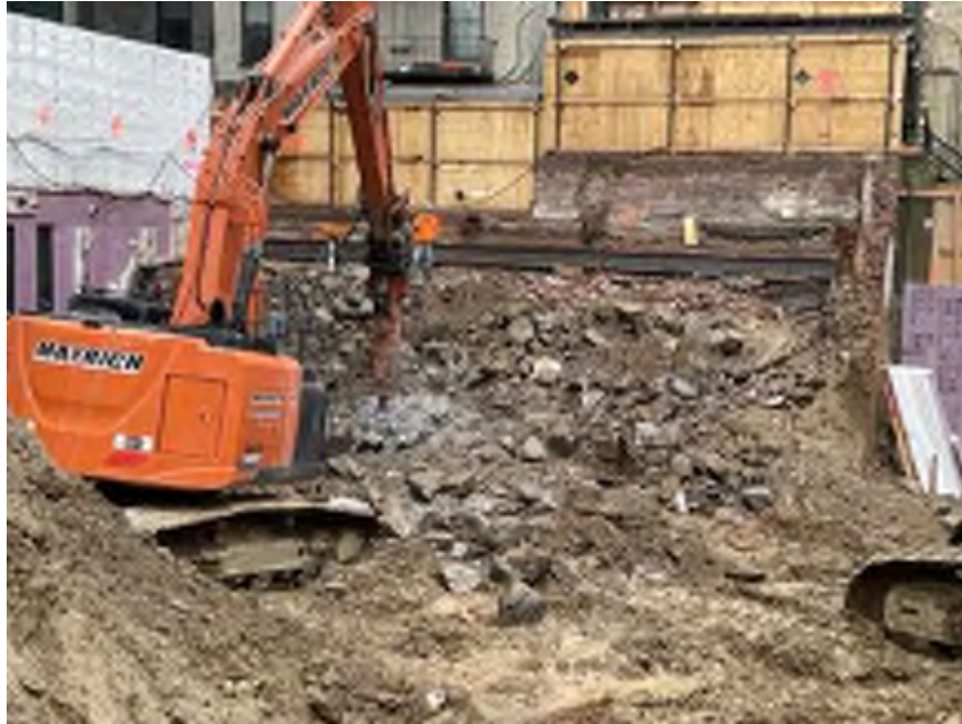
Photo 1: Mayrich applying dust suppression while breaking concrete in the southeastern part of the site (facing south)
