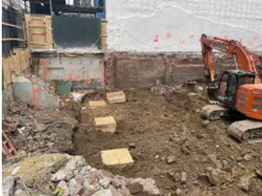
Photo 1: General view of non-hazardous historic fill and soil excavation on the northeastern part of the site (facing east)
