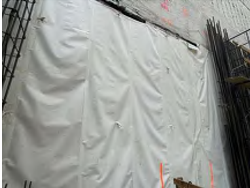
Photo 1: View of Mayrich installing waterproofing for the building's eastern foundational walls in the northeastern part of the site (facing east).
