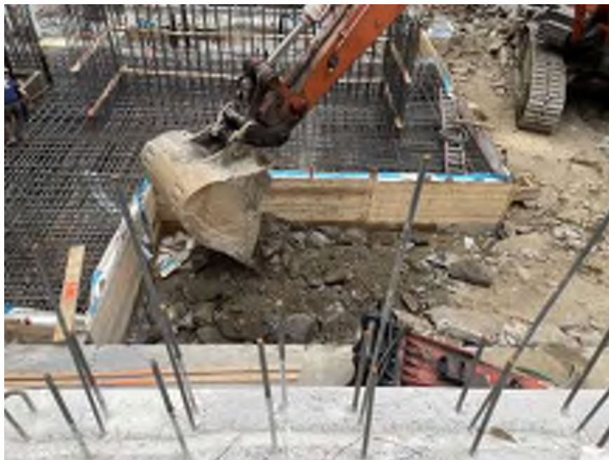
Photo 2: Mayrich temporarily backfilling with chipped bedrock to support formwork in the northeastern part of the site (facing south)
