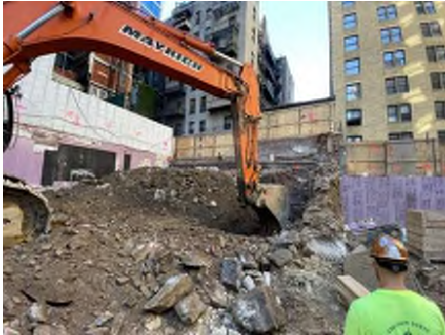
Photo 1: Mayrich excavating non-hazardous historic fill and C&D debris in the southeastern part of the site (facing southeast)
