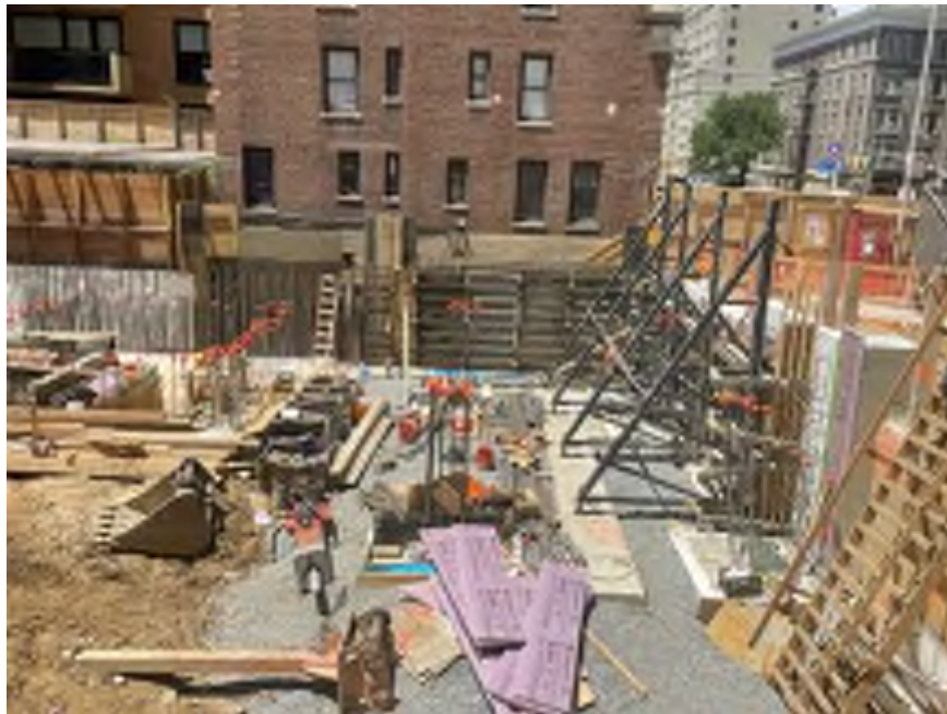
Photo 2: Current site conditions in the northwestern part of the site (facing west).
