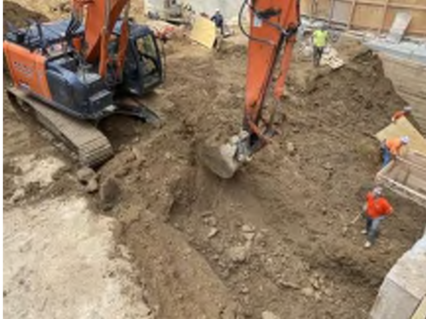
Photo 1: Mayrich excavating non-hazardous historical fill and native soil in the northwestern part of the site (facing southwest).
