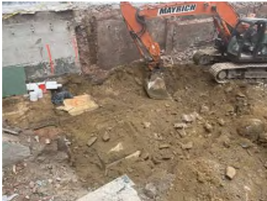
Photo 2: General view of non-hazardous historic fill and soil excavation on the northeastern part of the site (facing east)
