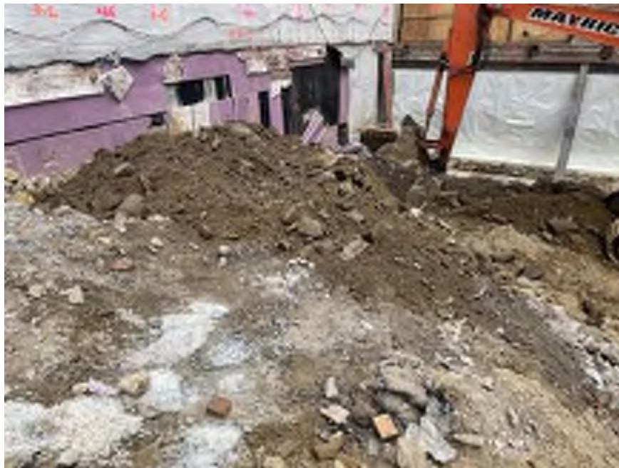
Photo 2: Mayrich excavating non-hazardous historic fill and chipped bedrock in the southeastern part of the site (facing south).
