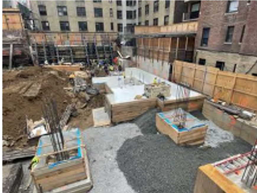
Photo 1: View of the area Mayrich backfilled with 0.75-inch stone in the northwestern part of the site, facing south.
