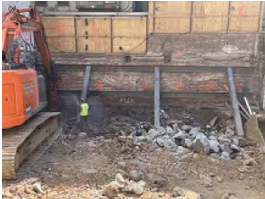
Photo 2: Mayrich using dust suppression while breaking concrete in the southeastern part of the site (facing south)
