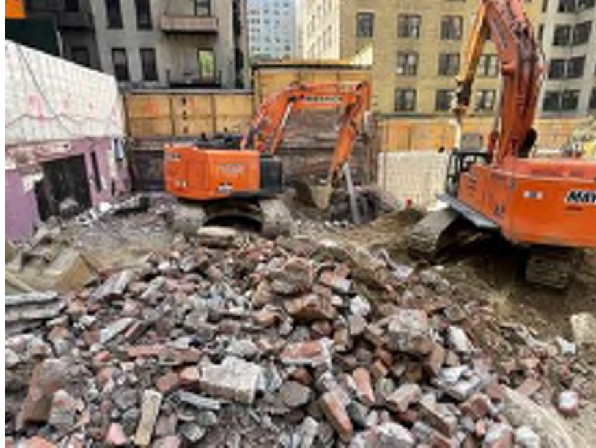
Photo 1: Mayrich removing C&D debris in the southeastern part of the site (facing south).
