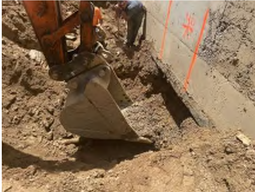
Photo 1: Mayrich excavating native soil along the western site boundary of the site (facing south).
