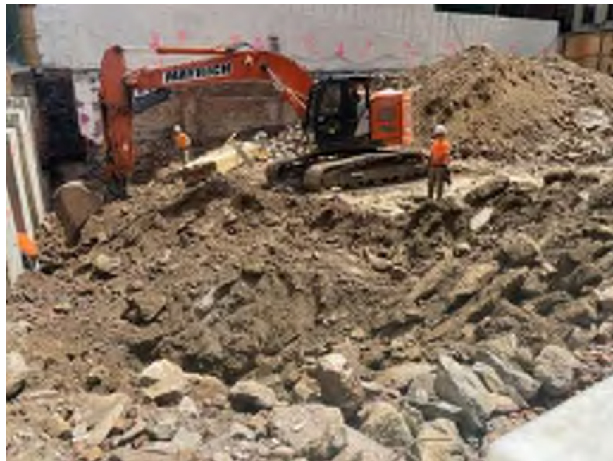
Photo 2: Mayrich excavating non-hazardous historic fill and native soil in the northern part of the site (facing east).
