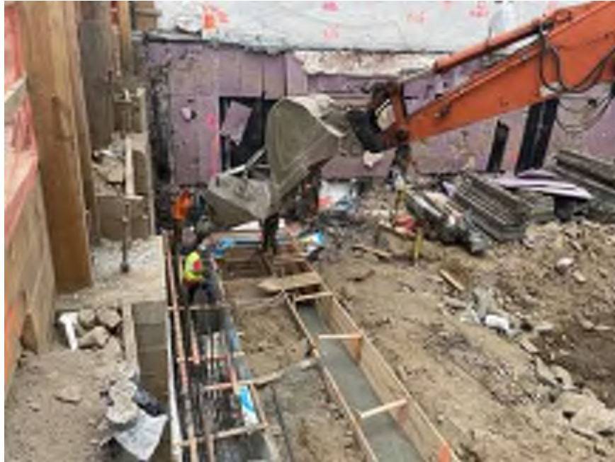
Photo 1: General view of Mayrich temporary backfilling around formwork frames with chipped bedrock and concrete in the northeastern part of the site (facing northeast)
