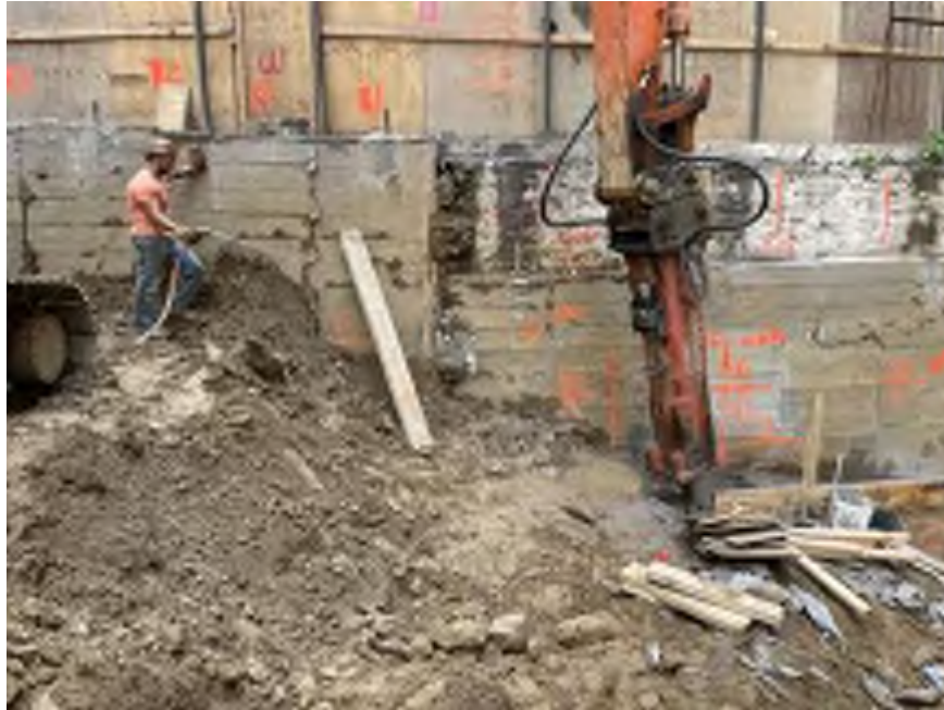
Photo 1: Mayrich applying dust suppression during bedrock chipping on the southwest part of the site (facing south)
