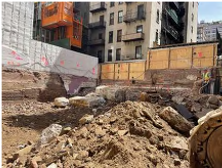
Photo 3: Mayrich applying dust suppression in the southern part of the site (facing southeast).
