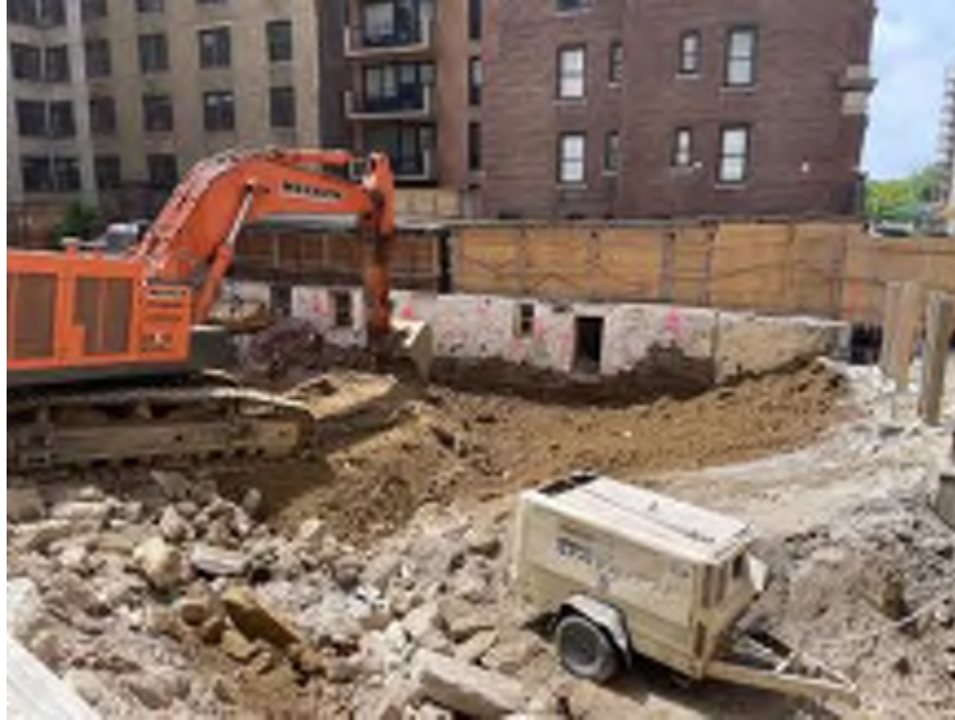
Photo 1: Mayrich excavating non-hazardous historic fill and native soil along the western part of the site (facing west).
