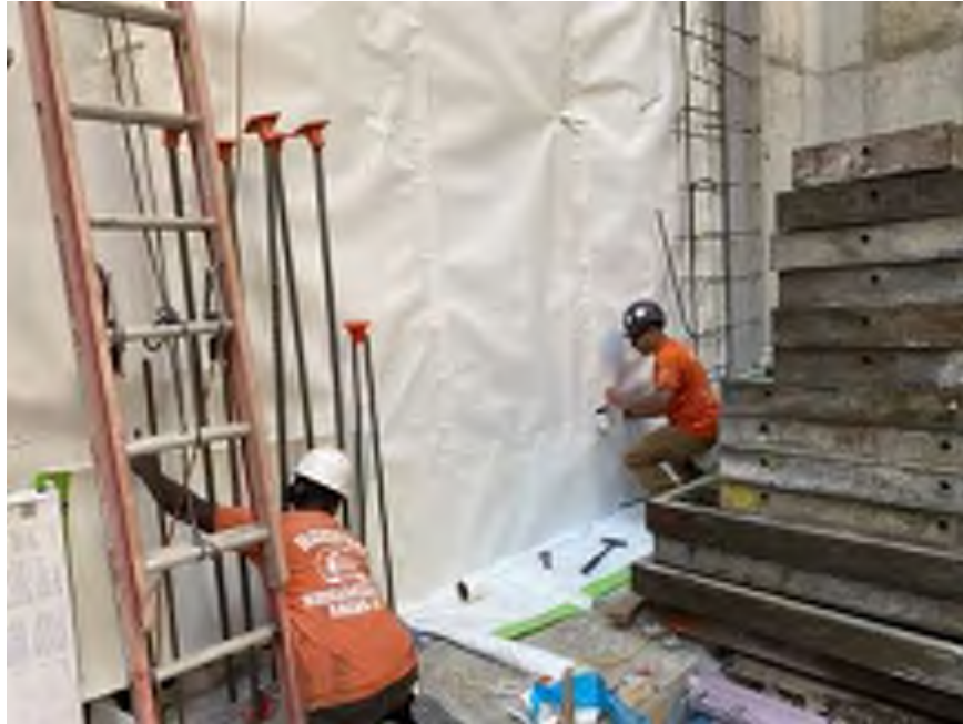
Photo 1: View of Mayrich installing waterproofing in accordance with manufacturer specifications in the eastern part of the site (facing east).
