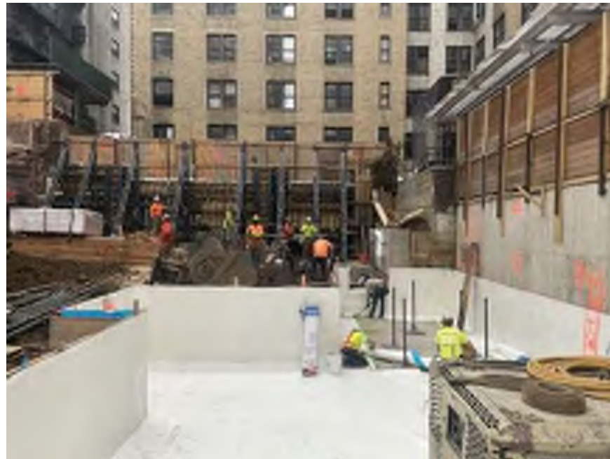
Photo 2: Mayrich installing waterproofing in the western part of the site (facing south)
