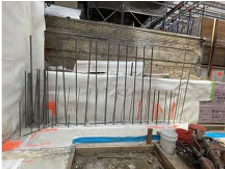
Photo 2: View of waterproofing installed along the southwest boundary of the site (facing west).
