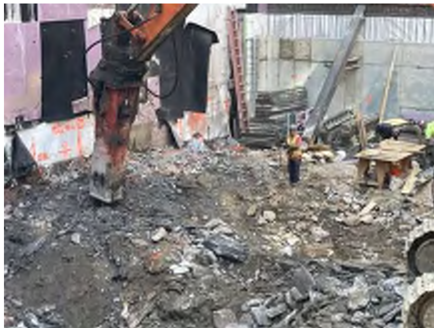
Photo 2: View of Mayrich using dust suppression while chipping bedrock in the southeastern part of the site (facing south).
