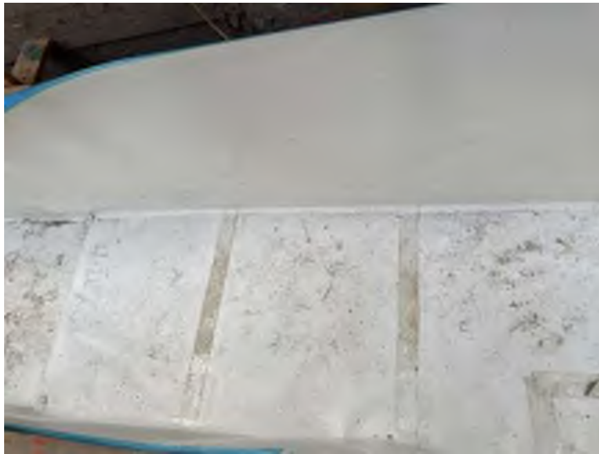
Photo 2: General view of waterproofing installed along the northern boundary of the site (facing north).
